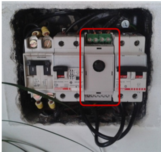
Figure 5.9: Installation of the APM in site #5. The red box highlights the device.
