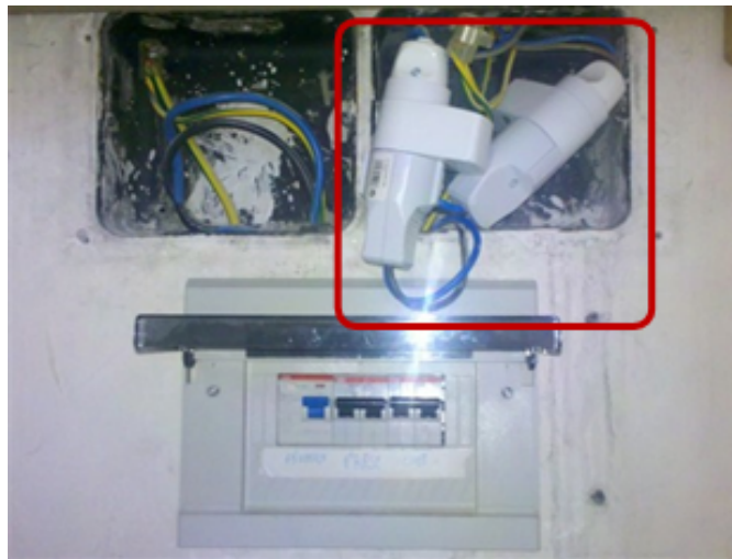
Figure 5.8: Installation of the Plugwise module in site #4. The red box highlights the modules.
